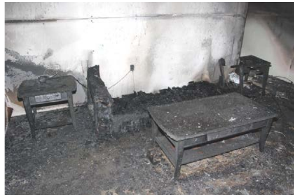
Figure 23: Post Fire Damage
