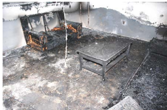
Figure 24: Post Fire Damage
